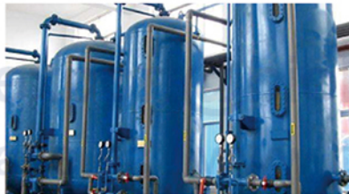
Boiler Softening Water
